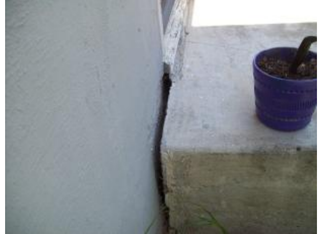
Example of one of the concrete stoops that has settled and pulled away from the building.
