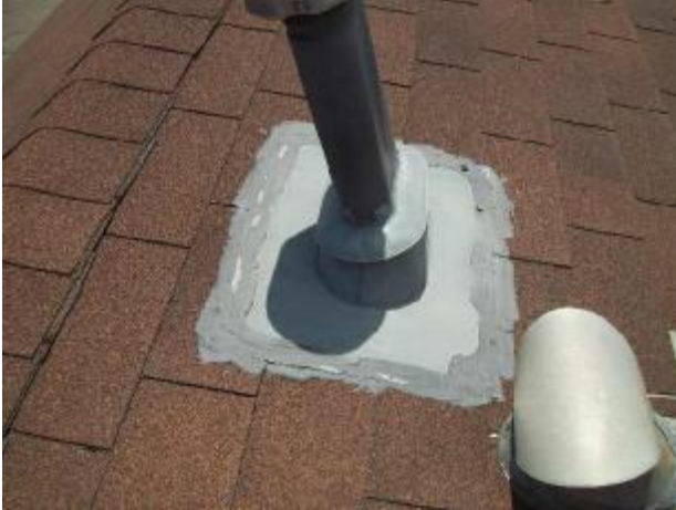
Improper flashing at the wall heater vent flue.
