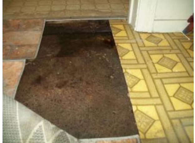
Moisture damage to the subflooring in the laundry room in Unit 124.
