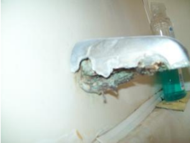
Corroded spout at the bathtub in Unit 124.
