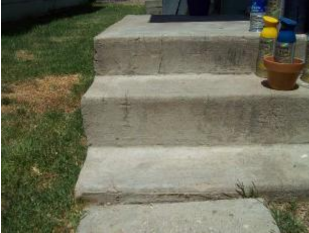
Example of the inconsistent riser heights at the front entry and rear entry concrete steps.
